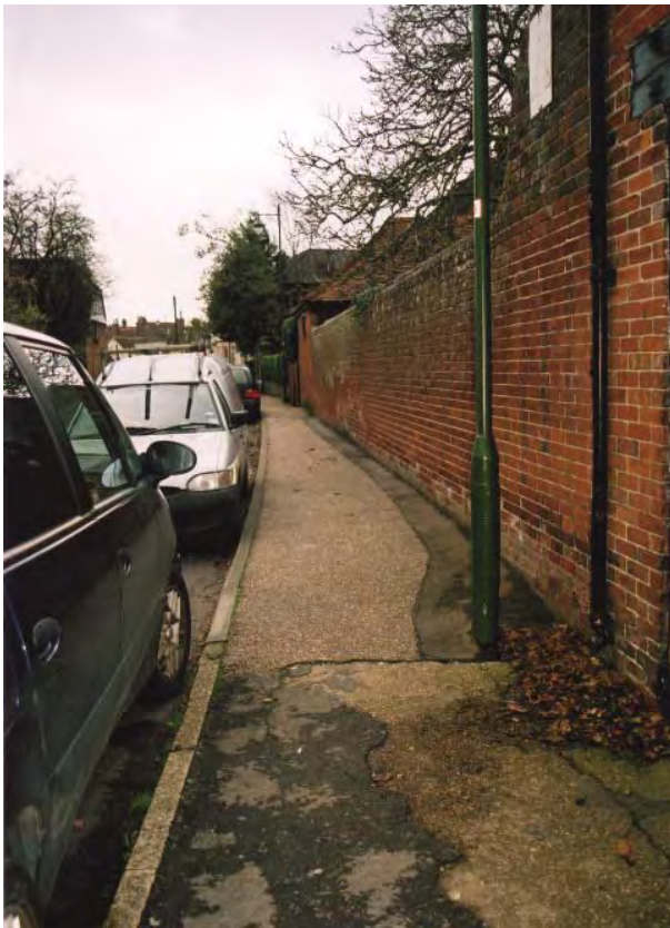
Poor quality pavements in North Street
